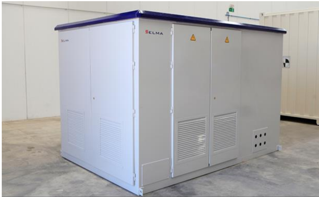
Plate 3-8: Typical transformer cabin (including switchgear)
