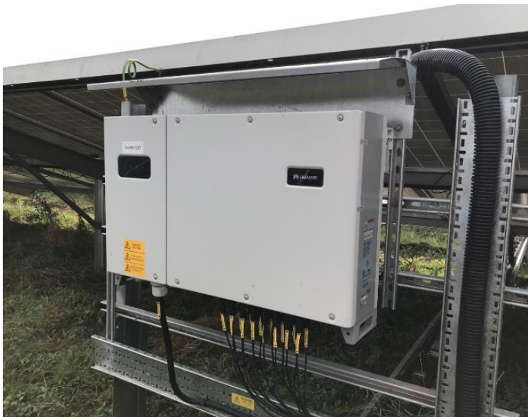
Plate 3-7: Typical string inverter
