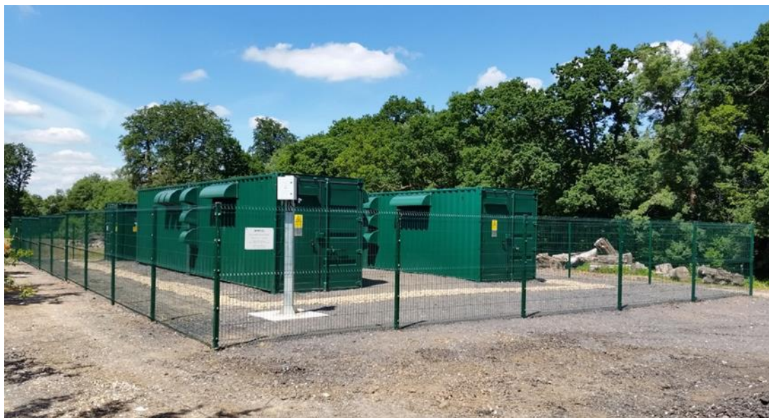
Plate 3-5: Solar Station Compound with Solar Stations Housed in Several Units
