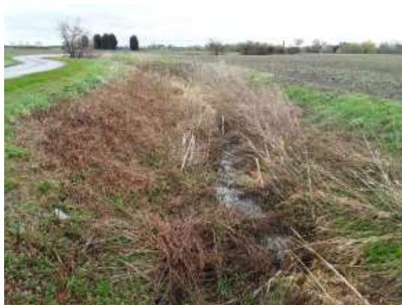
Photo 14 – Wet drain at TN33
